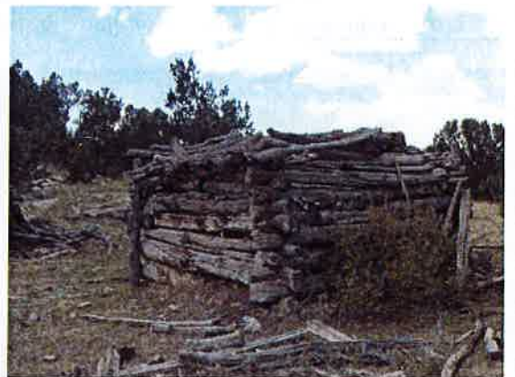
5LA.11695 Log buildings such as this one were rare within the survey area.
