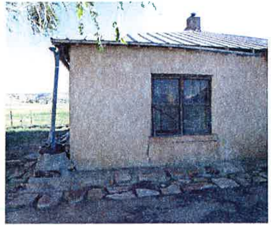
5OT.1104 Corner cistern
